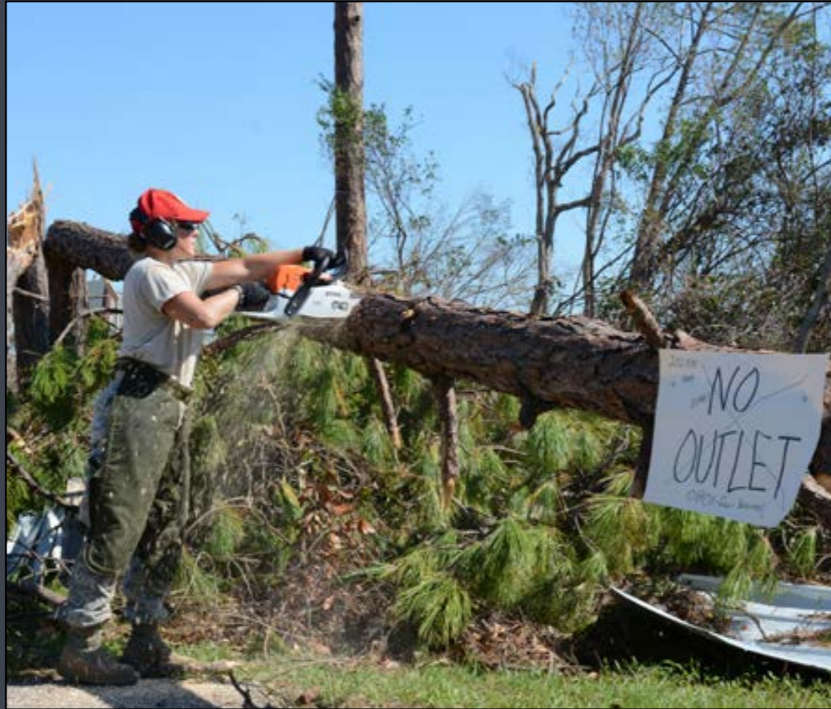
U.S. Air Force Staff Sgt. Colleen Curren, a structures journeyman with the 202nd Rapid Engineer Deployable Heavy Operational Repair Squadron Engineers (RED HORSE), chainsaws through a fallen tree on Debi Road in the Bayou George area of Panama City, Florida, Oct. 14, 2018, after Hurricane Michael. (U.S. Air National Guard photo by Staff Sgt. Carlynnne DeVine)
